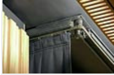
Detail of Triple E Chaintrack with acoustic curtain in Hall One at The Sage Gateshead
